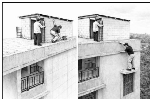
Figure 2. Observed work-at-height maintenance activity at approximately 10–12 m elevation without adequate fall protection systems
