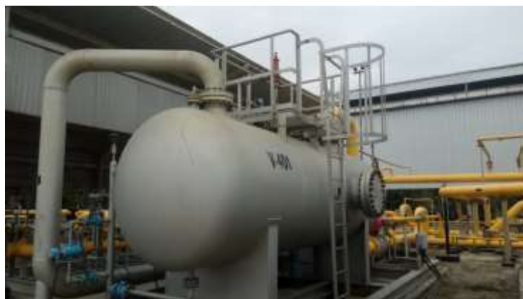
Gambar 1. Separator Horizontal 2 Fasa SGP 1 EMP Bentu Ltd
