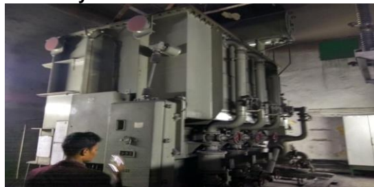
Gambar 13. Transformator Electrical Arc Furnace 6
